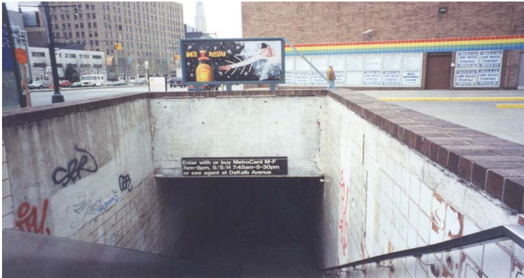
DeKalb Avenue station, Brooklyn (M/N/R/Q/Q Diamond). While this part-time entrance provides hour and MetroCard information, it lacks a station name sign with lines serving the station.
