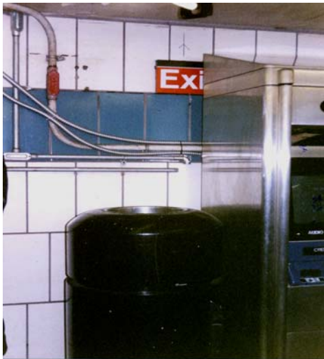
Fulton/ Broadway Nassau Street station, Manhattan (A/C/J/M/Z/1/2/4/5). TVM machine is blocking an exit sign.
