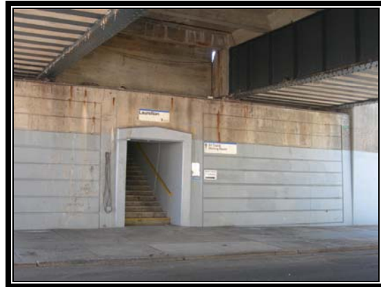
Poor Lighting in Underpass
