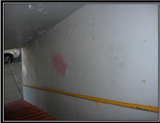
Graffiti in Poorly Lit Stairwell
